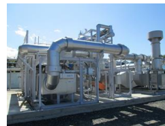
“K-FILTER” VOC emission treatment equipment
