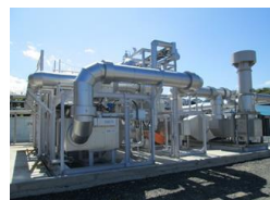
VOC emission treatment equipment
