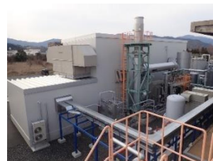
Gas cogeneration facilities at Tsuruga Research and Production Center
