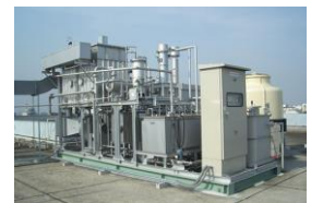
Equipment for VOC emissions treatment
