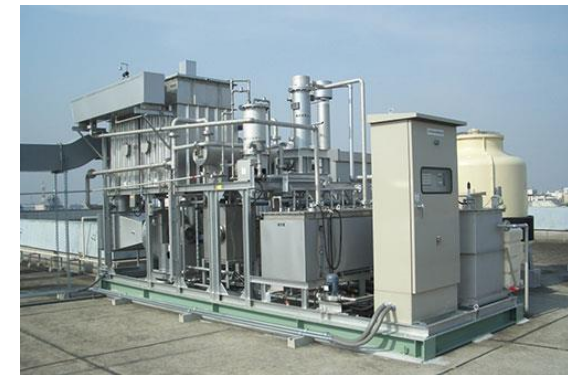
Equipment for VOC emissions treatment
