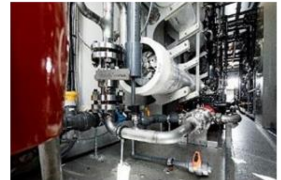
Salt Power's osmotic power plant
