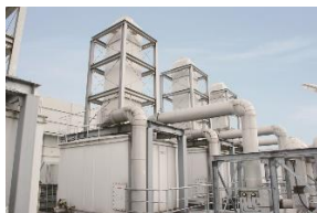
VOC recovery equipment
