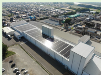
At the Inuyama Plant, 1,608 solar panels installed on the rooftop generate approximately 500 kW.
