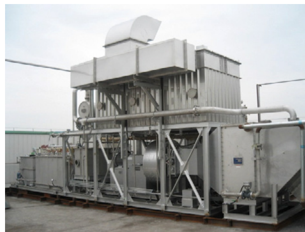
VOC recovery equipment
