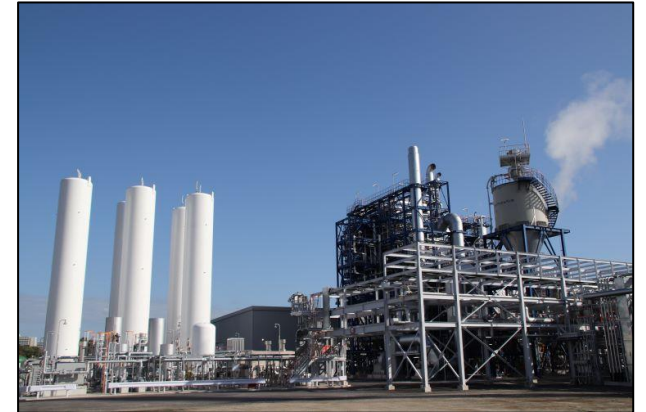
Newly constructed in-house thermal power generation plant at the Iwakuni Production Center
