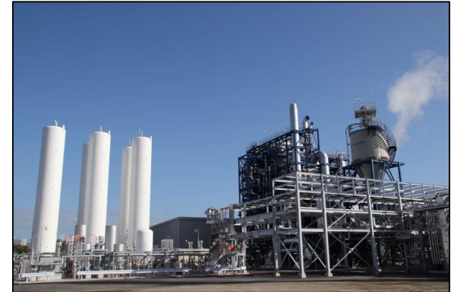
Newly constructed in-house thermal power generation plant at the Iwakuni Production Center
